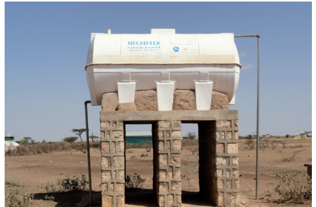
FIGURE 10 WATER STORAGE TANK
