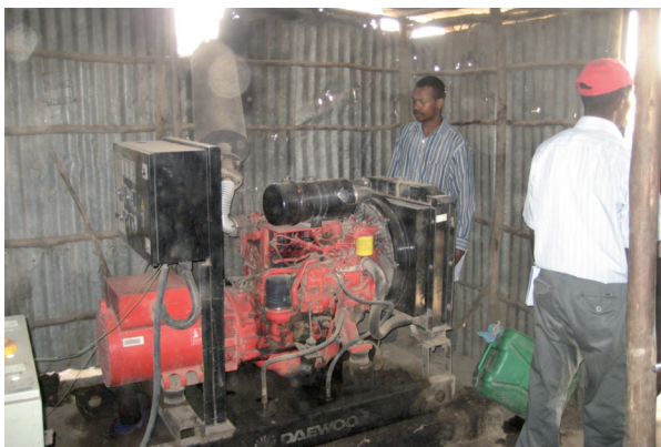
FIGURE 15 ELECTRICAL EQUIPMENT AND GENERATOR HOUSE
