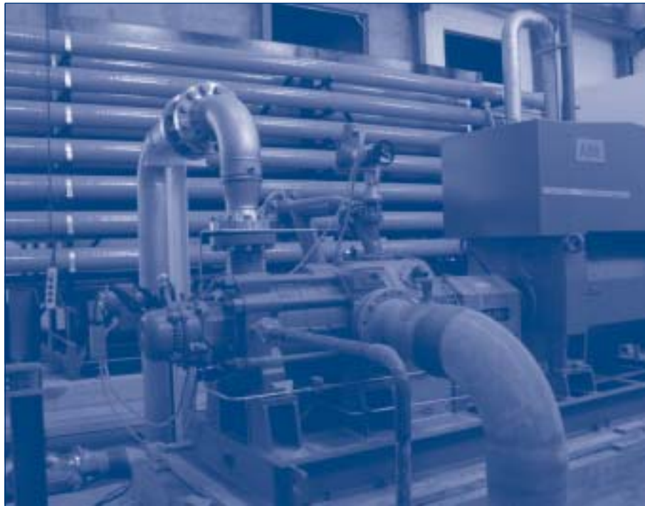
Fig. 18.11. Reverse osmosis (RO) racks and pump turbine system in La Aldea, Gran Canaria (capacity: 5000 m 3 /day; commissioned in 2001) (photograph by Jose M. Veza)
