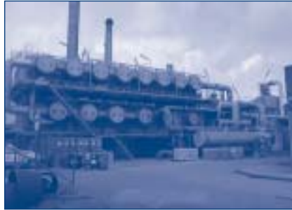
Fig. 18.4. Multi stage flash (MSF) distillation plant, Las Palmas, Gran Canaria (capacity: 2 \times 9,000 \text{ m}^3/\text{day} ; commissioned in 1980) (photograph by Jose M. Veza)
