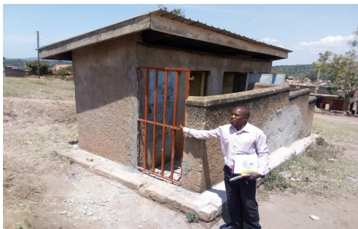
Picture of 2 stance pit latrine for girls Nwoya Central Primary school.
