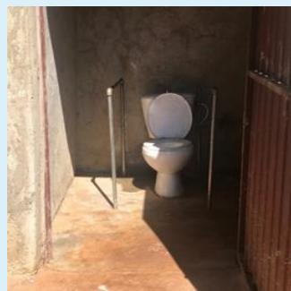
A health centre latrine in Bahir Dar Zuria woreda, Amhara region, with a well-made accessible cubicle on the left, including a good ramp, handrails and door opening to the outside. Inside there is a smooth entrance, enough space to move around, a raised seat, handrails and running water for flushing and washing.
