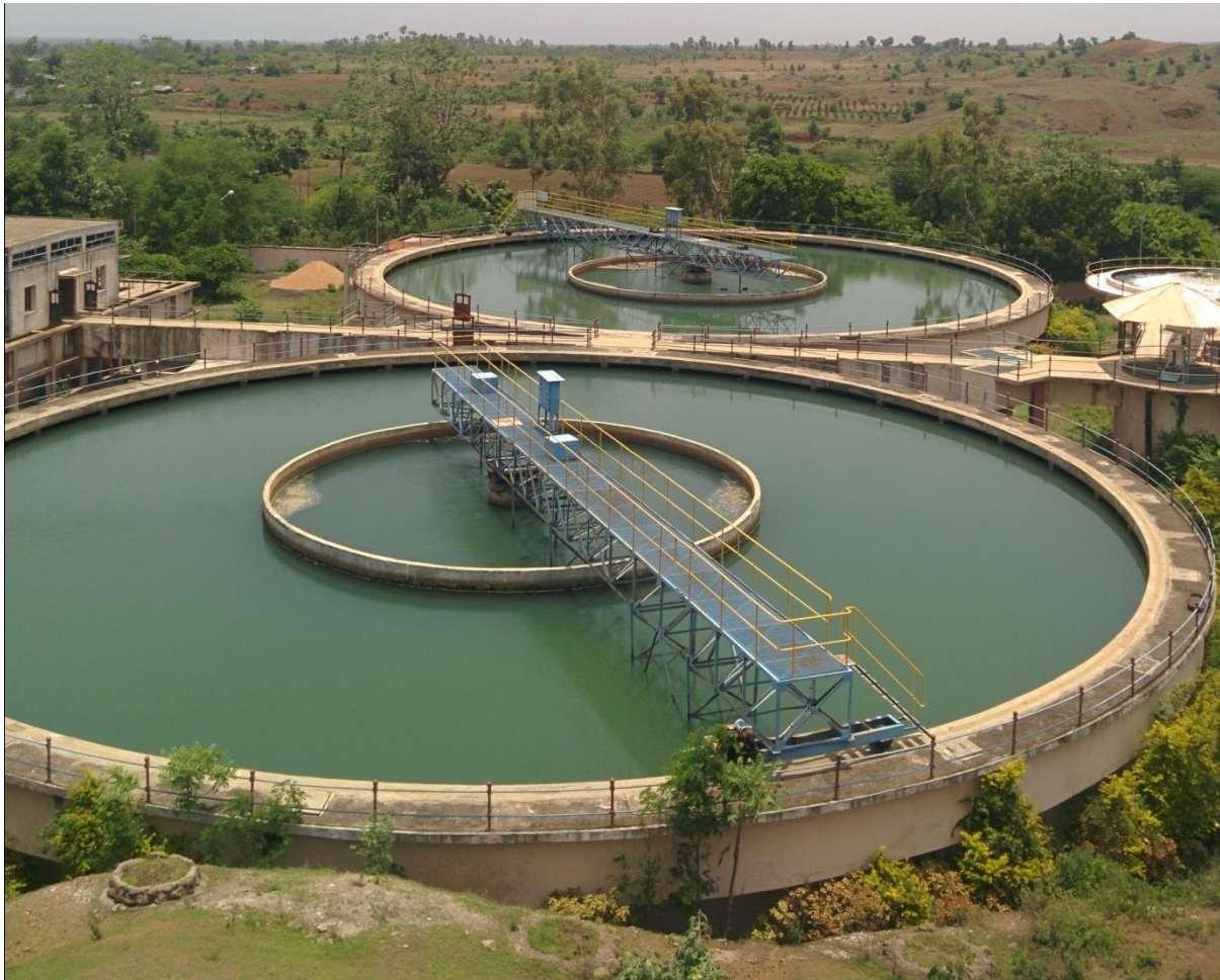
Photograph: Water Treatment Plant
