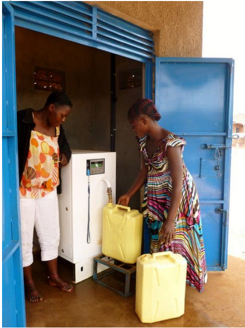
Figure 1: LIFELINK unit installed at Kikondo TradeWater business centre.
