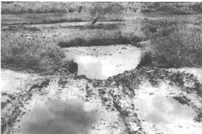
A burst sewage pipe near a WSP encourages mosquito breeding.
