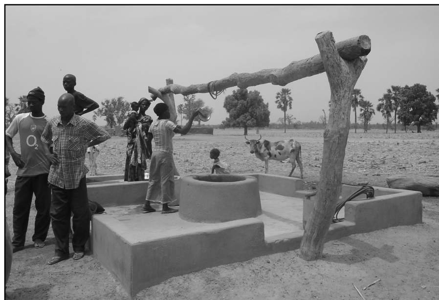
This medium-standard well has been lined and has a concrete surround
