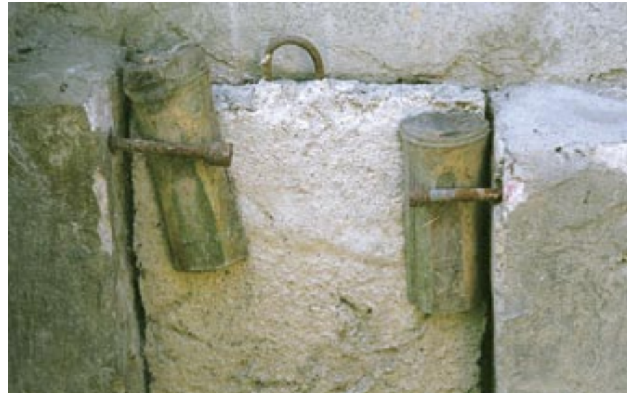
Example of vault doors with a simple locking system
