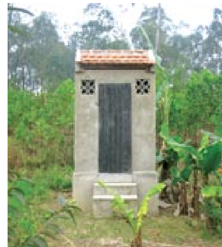
A DVC latrine in Tan Kim commune, Thai Nguyen Program Unit
