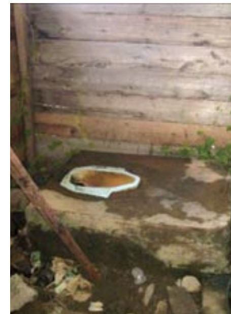
A typical toilet at a community centre in Aceh
