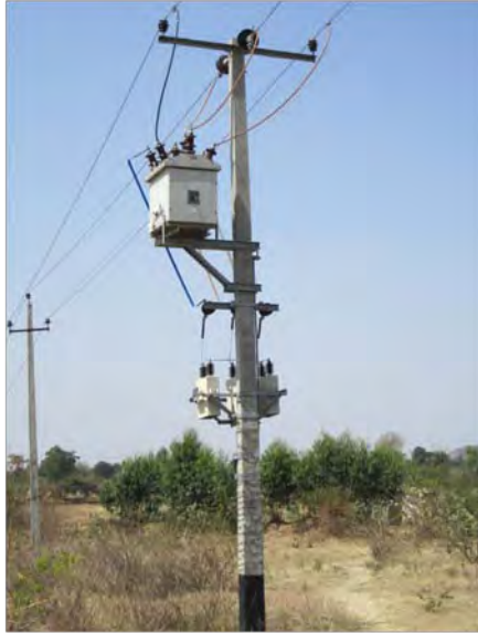
Capacitor, Doddaballapur Photo: K. Warr
