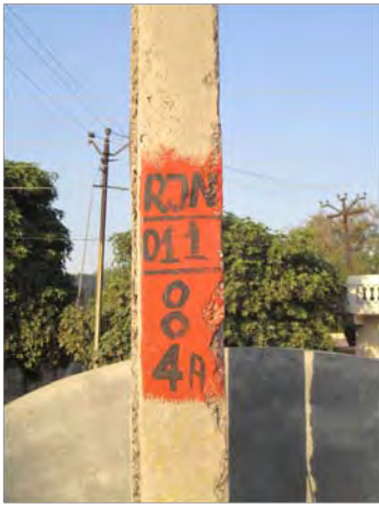
Each electricity distribution pole must have a unique number for the GIS system to function. Photo: K. Warr
