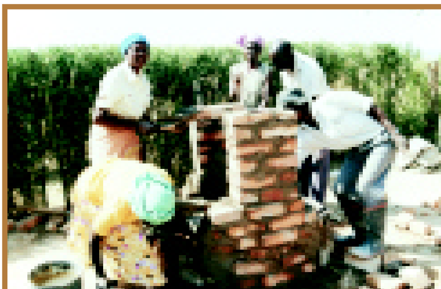
Upgrading a family well by building brick columns to raise the head works above ground level.
