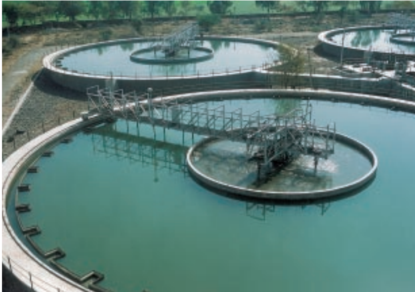
A filtration plant at Keki
