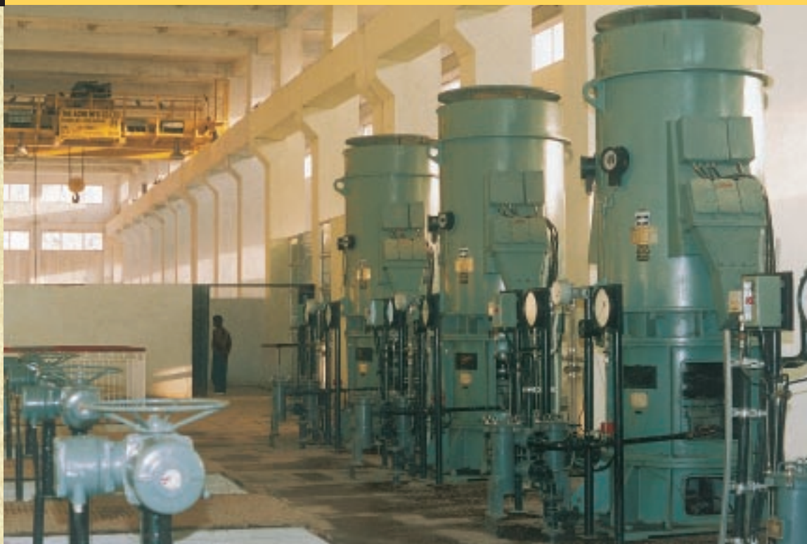
A privately maintained pumping station
