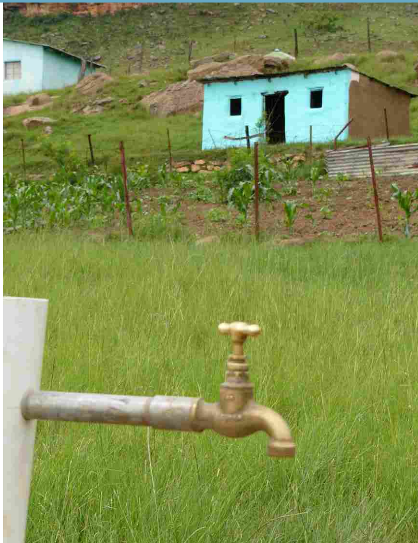
Municipal standpipe in Ukahlamba District Municipality, Eastern Cape
