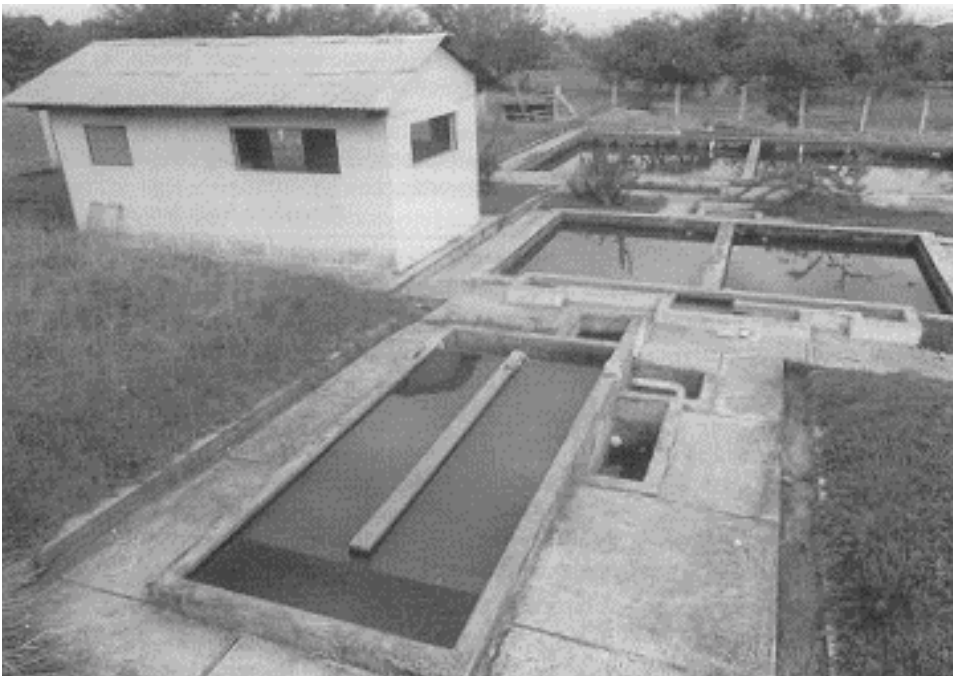
Figure 1: Multi-Stage Filtration plant in los Chancos, Valle de Cauca, Colombia
