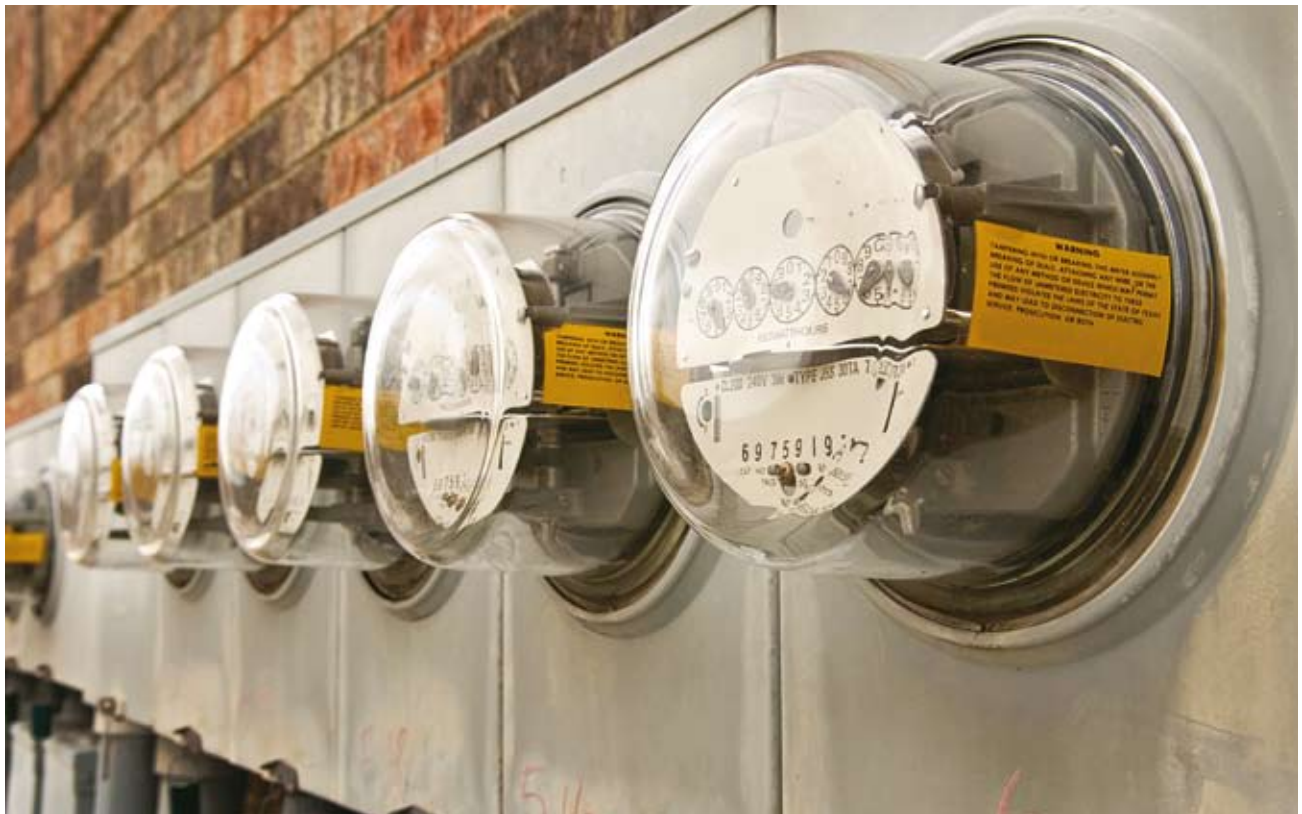
▲ Electricity meters in a city apartment building ©Wendell Franks/iStockphoto
