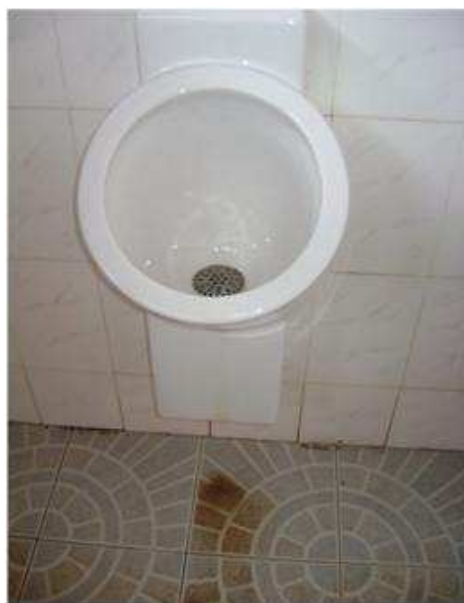
Figure 5-6 Waterless urinal at Valley View University
