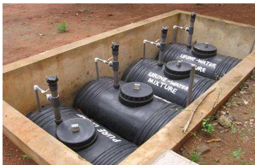
Figure 5-3: Urine Collection Tank at Valley View University, Accra, Ghana.
