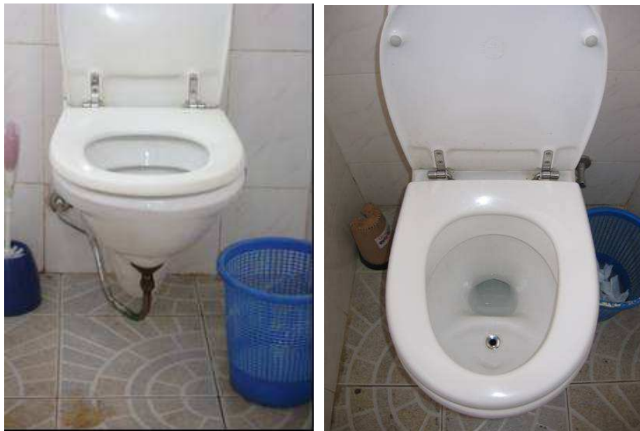
Figure 5-2 Urine diverting toilet at Valley View University
