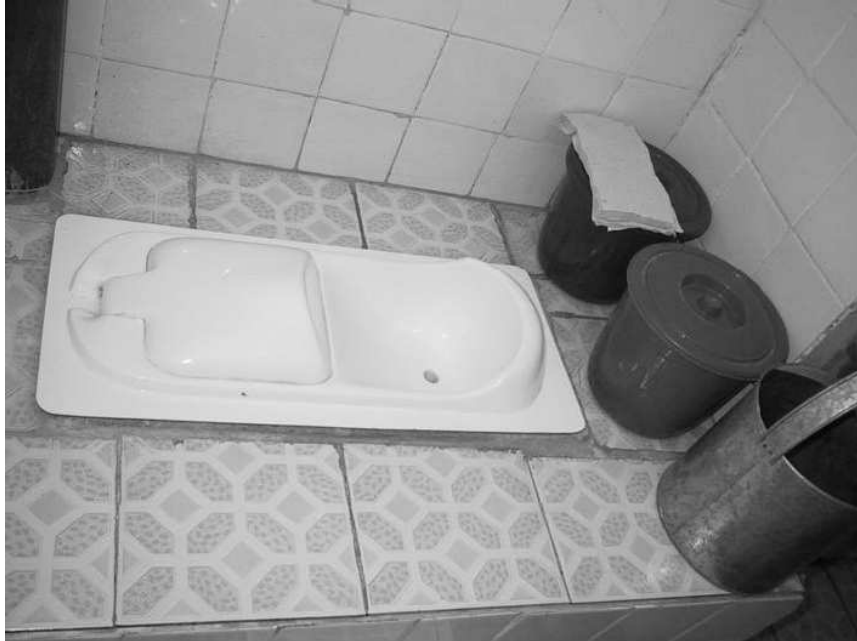
Figure 5-4 Harvesting of urine using a squatting closet (Dragnet, 2003)
