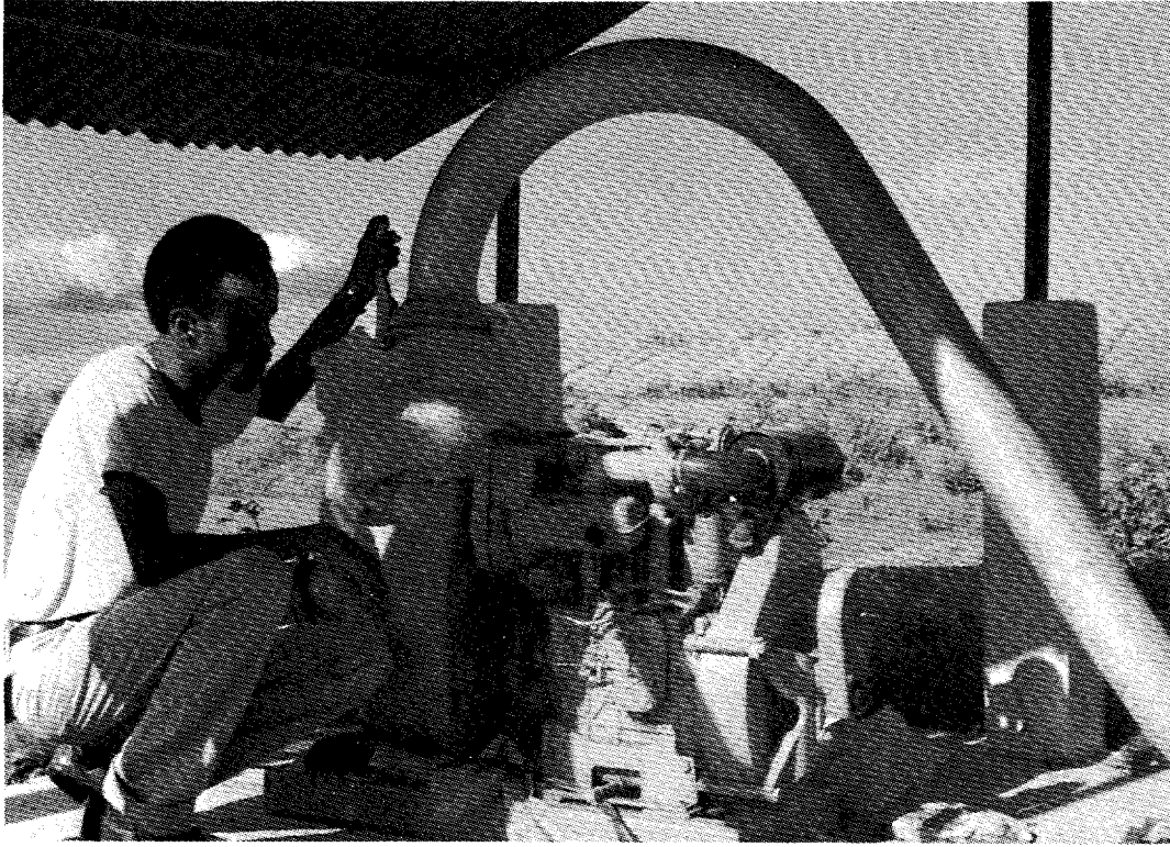
Diesel engine pumping system in Somalia.
