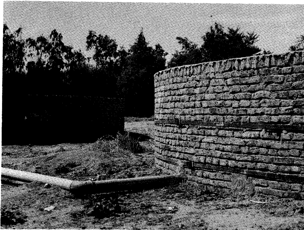
A storage tank adds considerably to the costs of a pumping system. The tank on the left has cracks in the outer wall. The tank on the right has been reinforced with steel straps.
