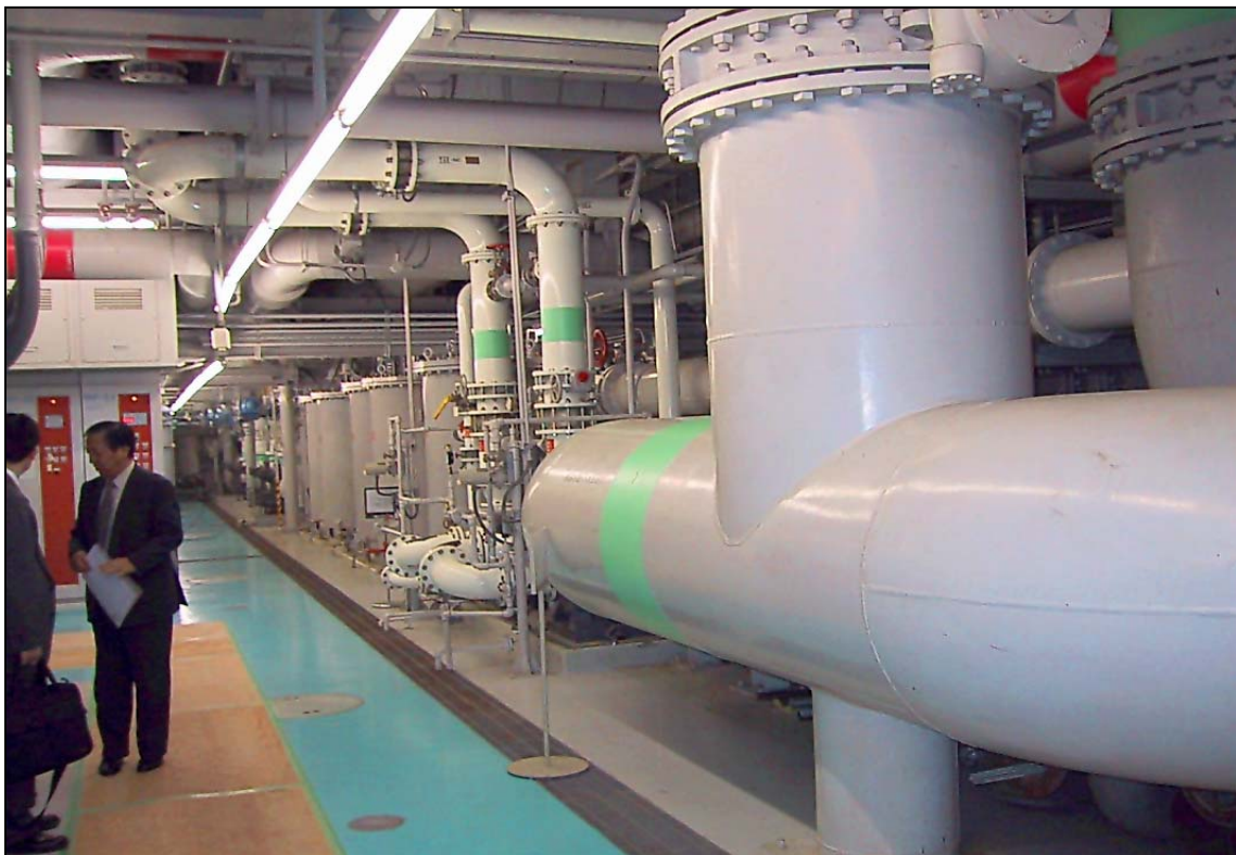
Figure 8: Chiba Service Water System (Photo: Rudolph, 2001)
