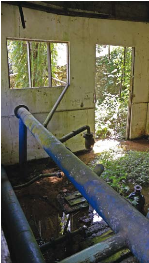
During the conflict, many REGIDESO centers, such as the above Ndjongobono station in Lisala, Equateur Province, were pillaged
