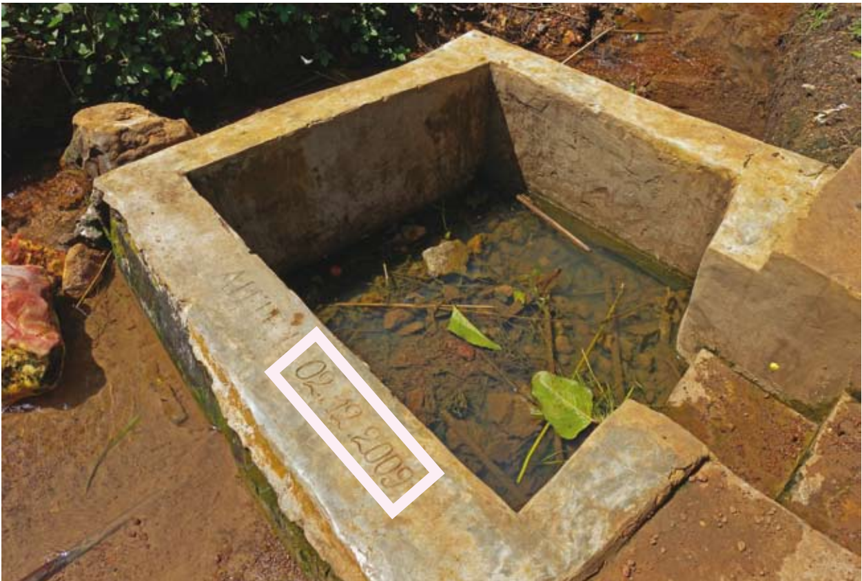
Constructed as recently as February 2009, SNHR advised that this poorly designed spring box in Boka village (Bandundu Province) be demolished as it posed a health risk to the local population
