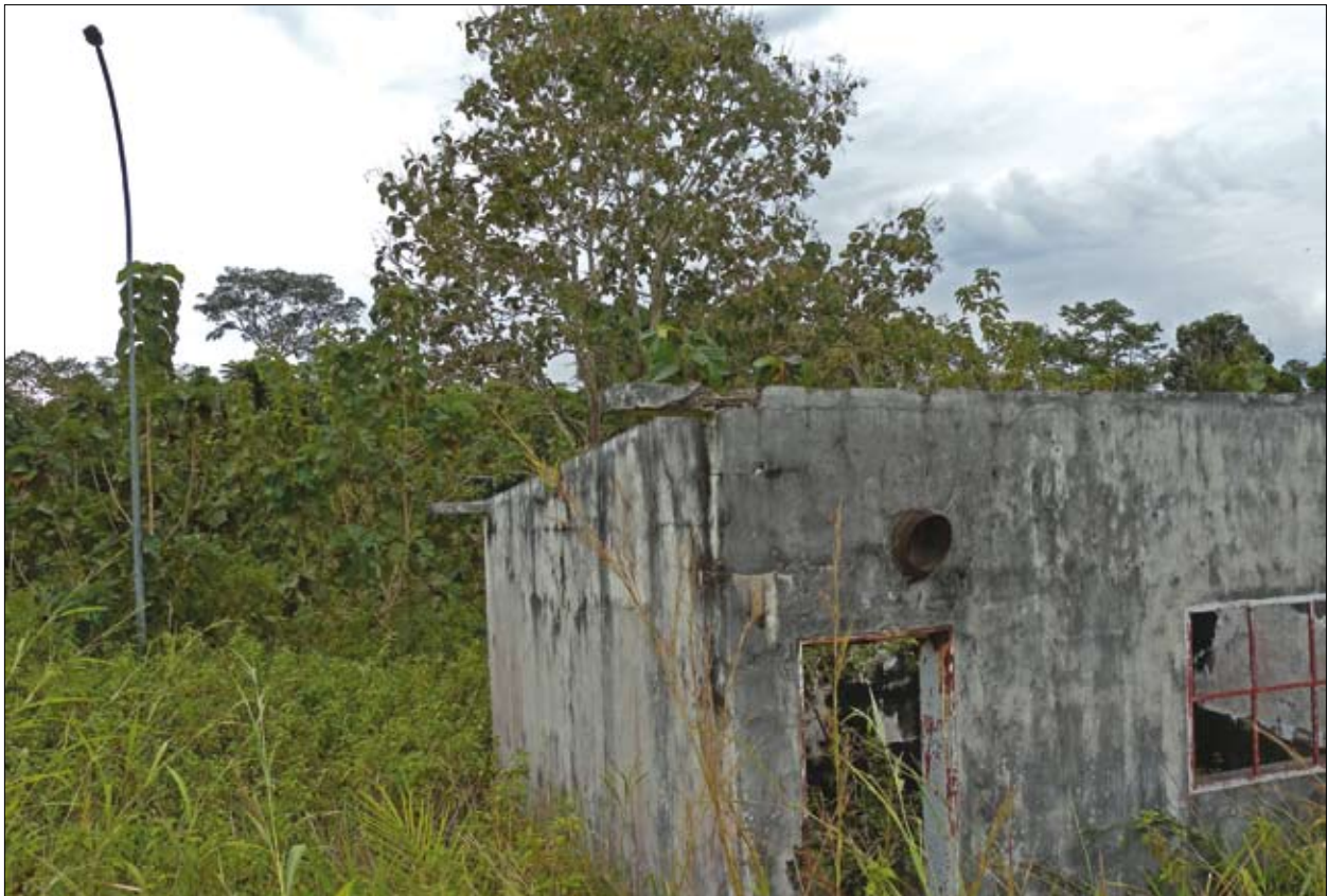
Abandoned in the early 1990s, the REGIDESO center in Libenge is overtaken by the forest. A lamp post relic points to the installation
