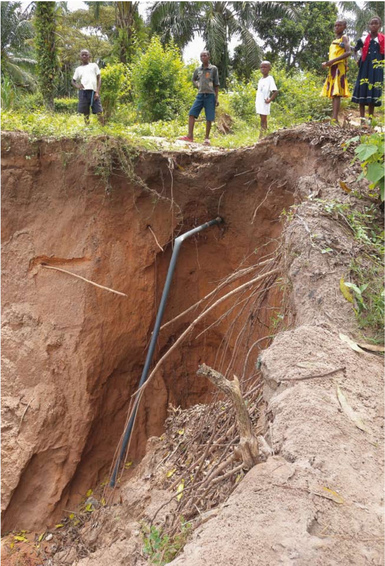
Gully erosion has damaged Kananga's water pipelines
