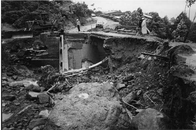
Figure 2: The Orosi bridge in Costa Rica collapsed under intense rainfall in 2002
