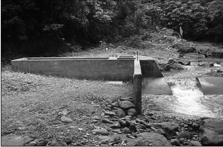
Figure 3: Gongolona, water intake (UCR study 2002)
