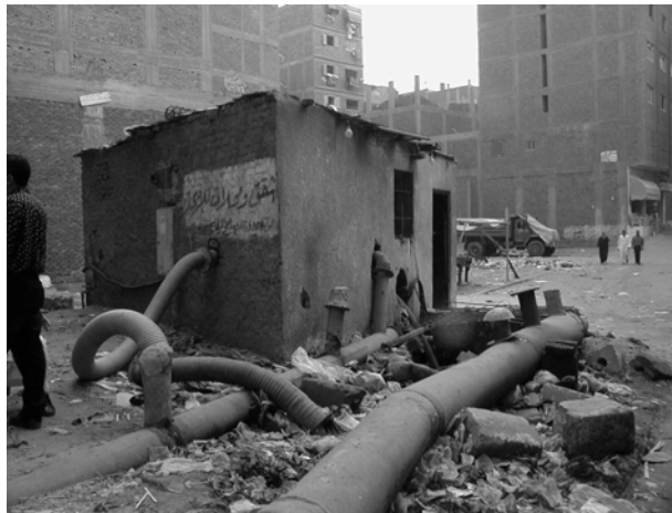
Temporary pump station in Ezbet el Nawar
