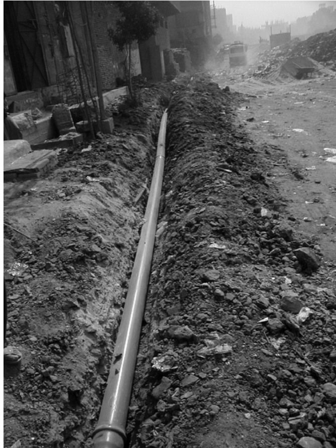
Installation of new 6" water pipe next to road bed. Note absence of sand bedding and shallow depth.
