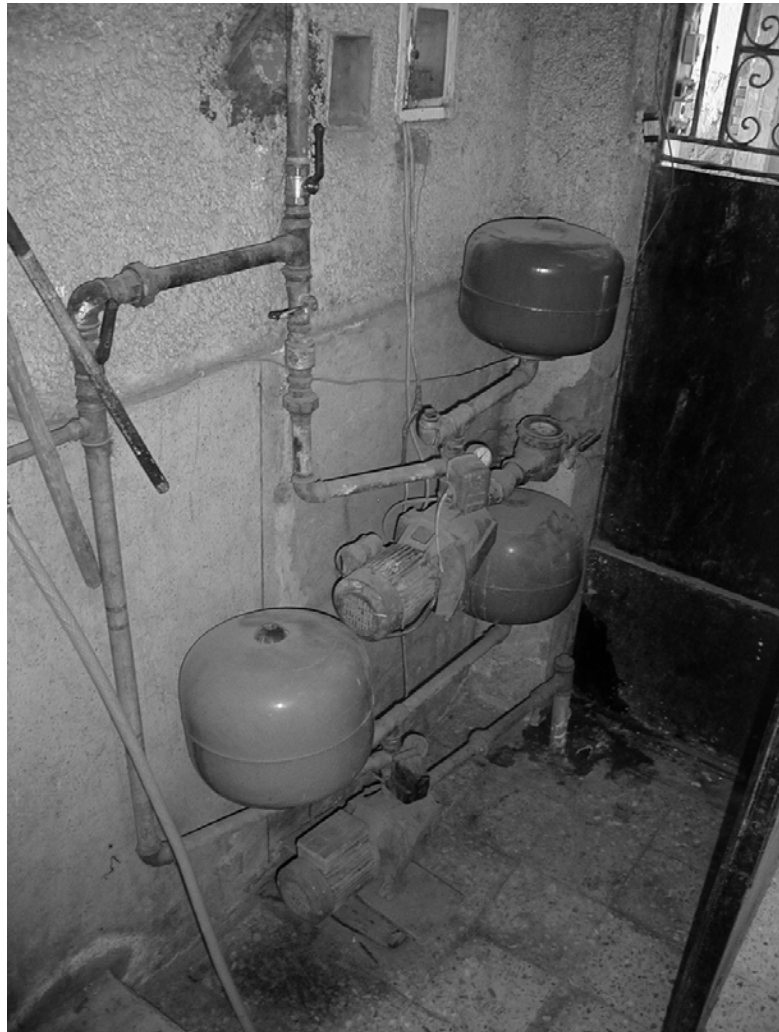
Cross connection between well source (lower line) and municipal water source with meter (upper).
