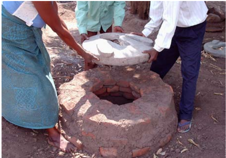
Installing small slab on bring ring beam for Arborloo Photo Credit: Peter Morgan
