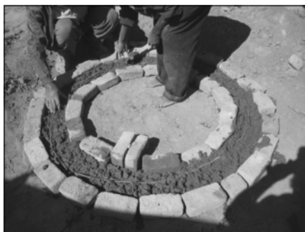
The concrete ring beam is being molded between two brick circles, and reinforced with wire.
