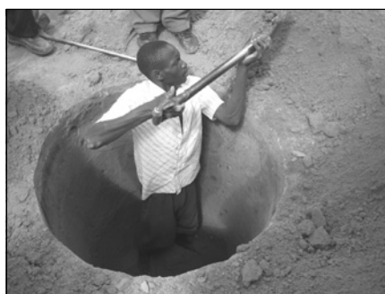
Once the ring beam has been made, the pit can be excavated beneath it.
