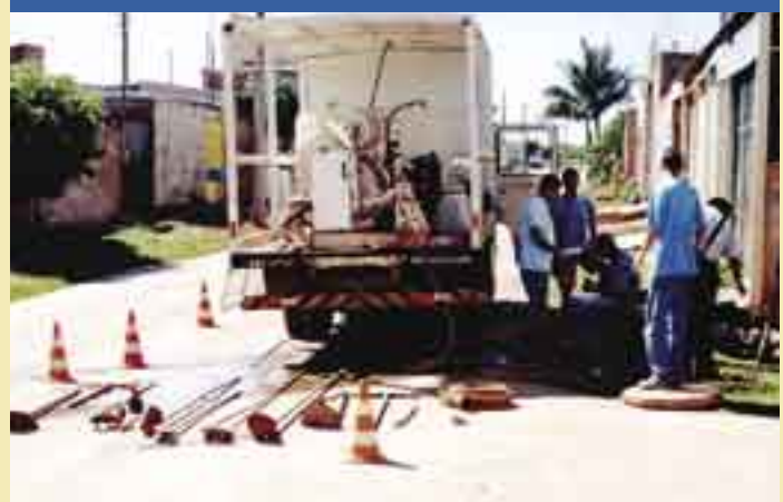
Maintenance Equipment for Condominal Branches, Brasilia
