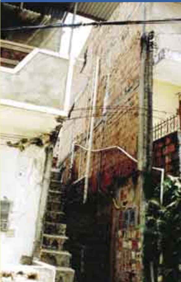
Sewerage pipe attached to wall, Sao Caetano, Salvador de Bahia
