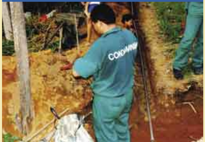
Intersection of Condominial Water Branch, Parauapebas
