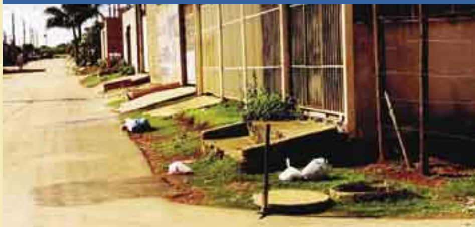
Condominial Box (seen open in the right hand lower corner), Riacho Fundo, Brasilia
