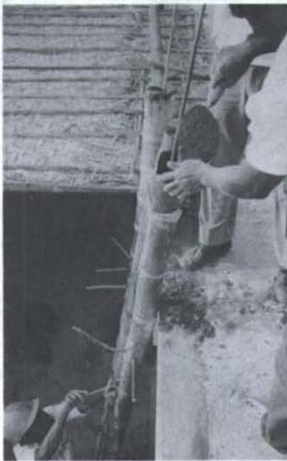
Reinforced concrete columns were cast inside hollow bamboo poles for the building supports.
