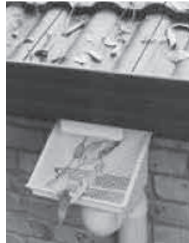
Screen over a downpipe
