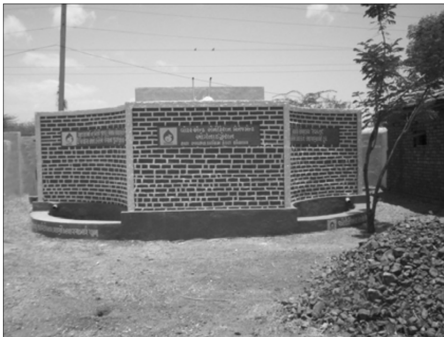
School sanitation corners proved an effective entry point for launching project activities while providing much-needed facilities.
