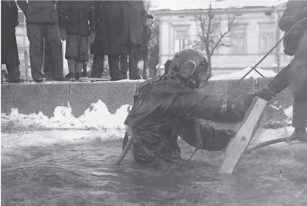
Plate 8. Diver installing water intake pipe in icy Lake Katumajärvi in February 1955 in Hämeenlinna, Finland (Photo: Hämeenlinna Regional Water and Sewage Company)
