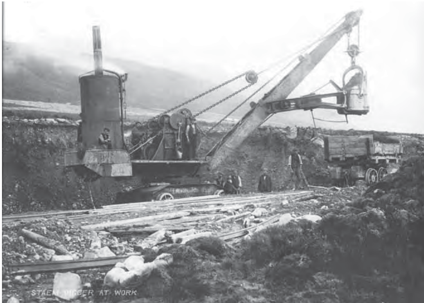
Plate 64. Steam excavator used for Talla Reservoir construction 1895–1905, South of Broughton / Peebles for water supply of Edinburgh, Scotland (Photo: Scottish Water)
