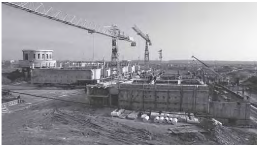
Plate 47. A new water treatment plant under construction in Bucharest, Romania in 2004 (Photo: Apa Nova Bucharest)
