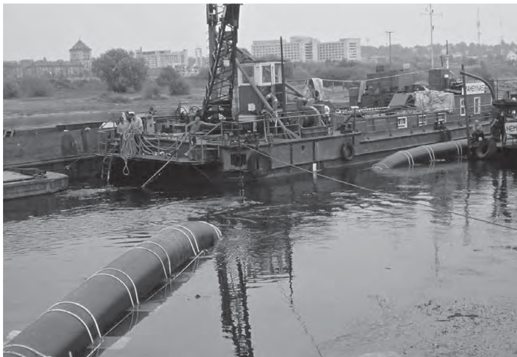
Plate 34. Laying of a submersible plastic sewer for Kaunas, Lithuania (Photo: P. Pietilä 1998)
