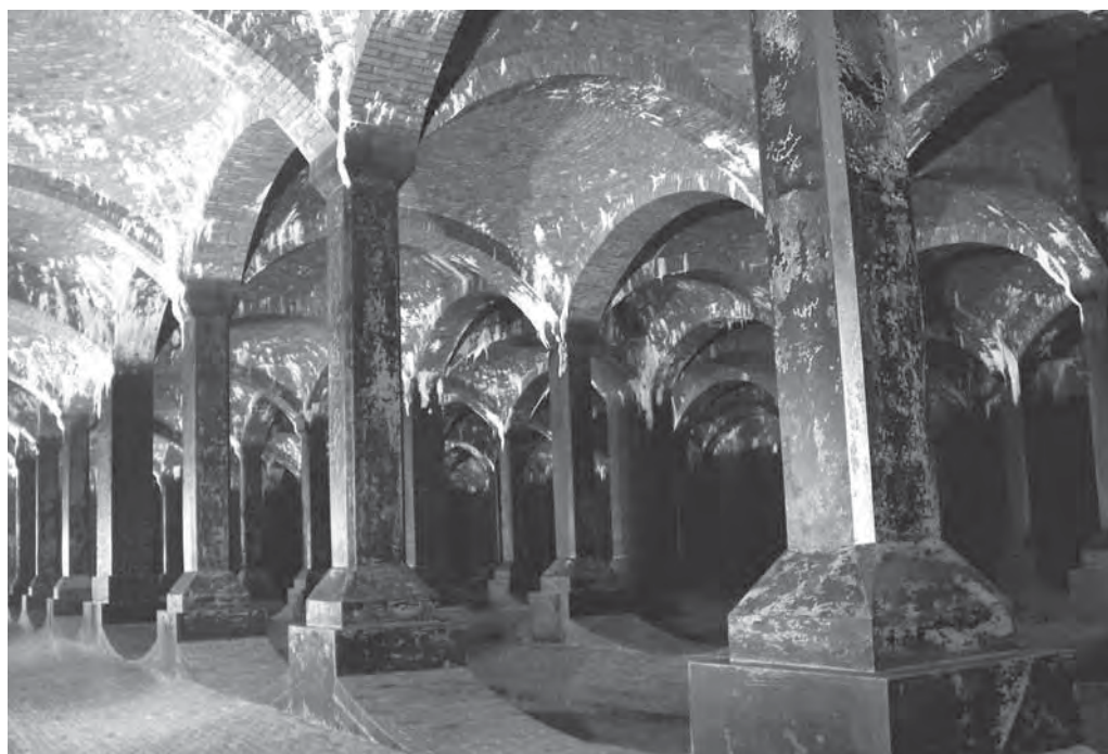
Plate 43. Inner view of the potable water tank of Łódź, Poland during conservation before filling with water, constructed originally in 1937 (Photo: Company of Water Supply and Sewage Systems in Łódź, ZWiK, 2002)
