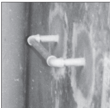
Figure 9.144. Handrail cemented to the wall.
