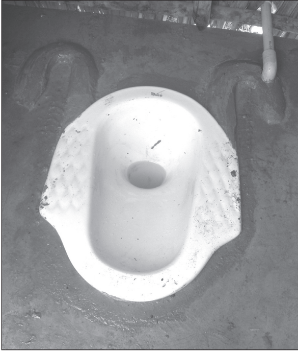
Figure 7.42. Cement mortar mouldings next to toilet pan for wheels of wheelchair to slot into for accurate positioning.
