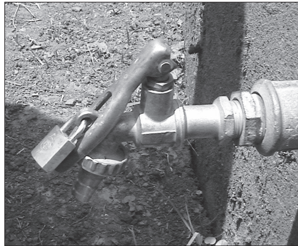
Figure 6.22. Lever operated tap with padlock. Unsuitable for a person with limited grip or stiff fingers. (Case-study 9.21, page 219)
