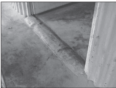
Figure 9.24. Flood prevention threshold has been rounded for easier wheelchair access.
