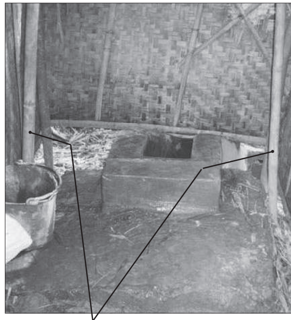
Figure 7.11. Two vertical bamboo support poles one on each side of latrine. (Case-study 9.9, page 183)
