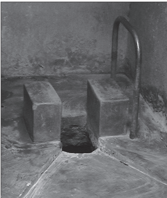
Figure 7.26. Twin cement-plastered brick sitting blocks. Height: 25cm; gap: 14cm. The gap makes anal cleansing easier than on an ordinary seat. (Case-study 9.26, page 232)
