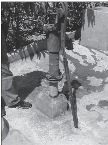
Figure 9.14. Water drains away from the apron.
