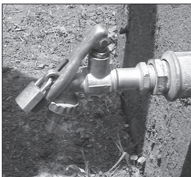
Figure 9.102. The tap can be padlocked.
