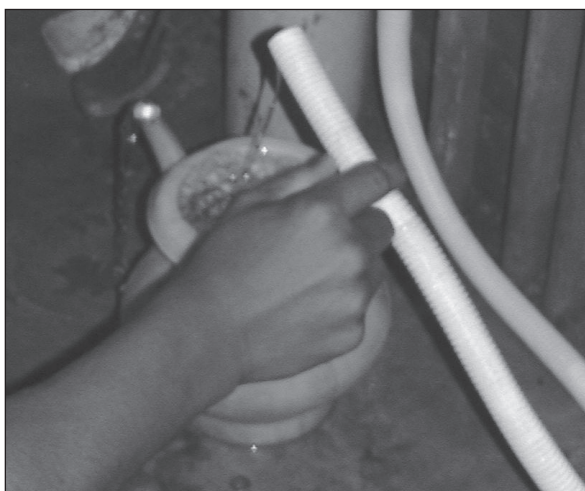
Figure 7.54. Flexible hose attached to a tap allows the user to fill a container with water using only one hand. (Case-study 9.6, page 177)
