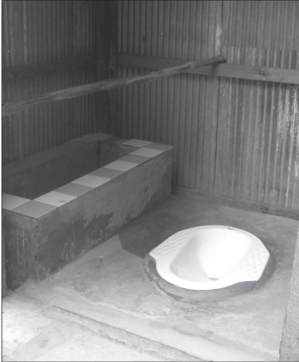
Figure 7.6. Single horizontal wooden rail (H: ~50cm) from door to back wall, for support to enter toilet. Too high for child to hold while squatting.
