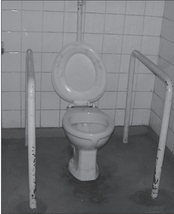
Figure 7.2. Painted handrails cemented to floor on both sides of pedestal toilet. 50mm Ø g.i. pipe; H: ~80cm.
