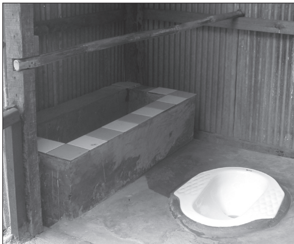
Figure 7.53. Water trough inside toilet cubicle. (Case-study 9.19, page 215)
