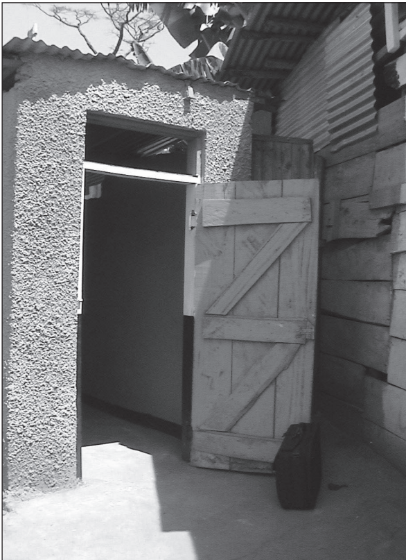
Figure 5.20. Toilet door with a two-way hinge allows this door to open outwards and inwards. Note the international disability symbol on the door.
