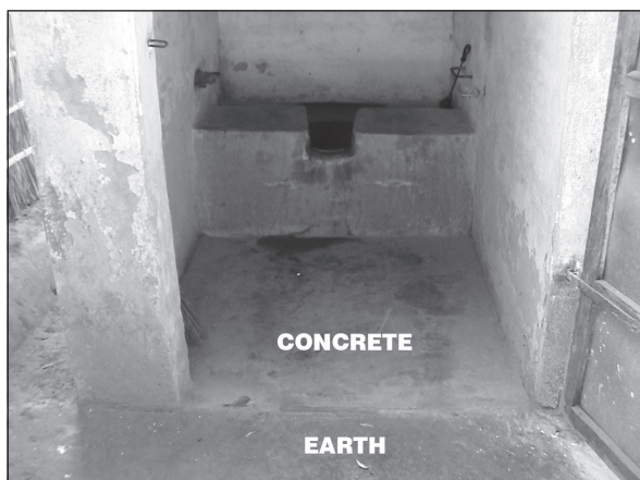
Figure 5.16. Toilet entrance. (Case-study 9.1, page 154)
