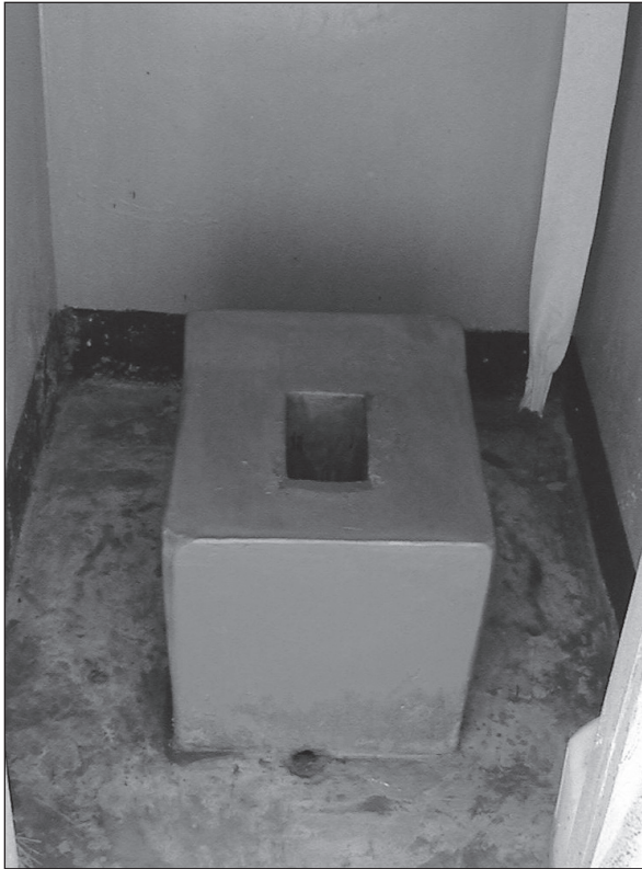
Figure 7.24. Toilet seat made of bricks, plastered with cement mortar and painted. Raised at the back for extra support. (Case-study 9.24, page 224)
