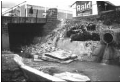
Industrial wastewater flows straight into a tributary of the Nairobi River
