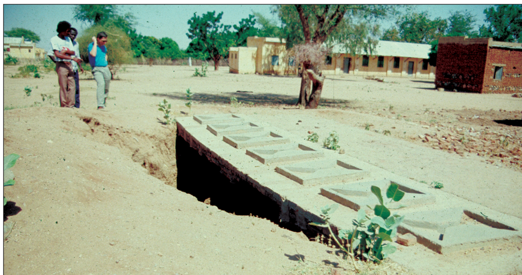
Failed unlined trench latrines, Sudan
