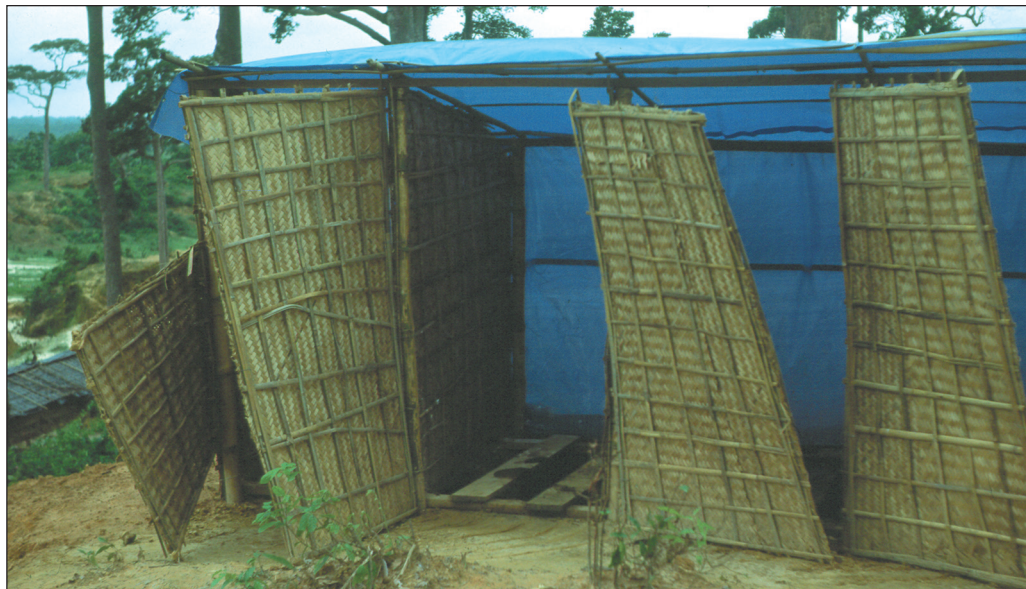
Simple trench latrines, Bangladesh
