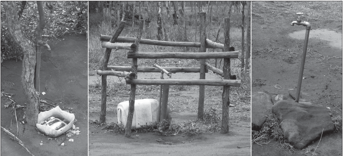
Figure 4 Standpipes without proper support structures. The standpipe in the middle shows an impromptu enclosure to protect the tap from domestic animals
