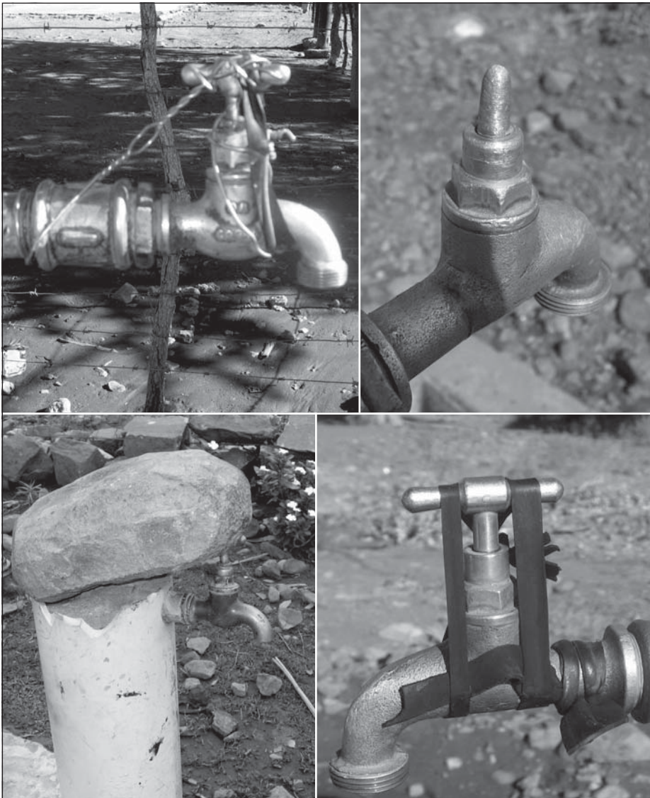
Figure 9 A tap with a worn-down stem (top right) and three ways to block a tap with a stripped stem – by binding it with wire, with elastic rubber strips and by keeping the stem down with a stone
