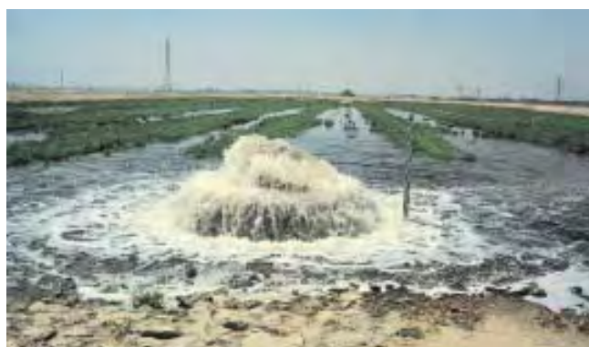
Pumps transfer water from the withdrawal wells to irrigation zones in the Negev Desert, Israel. Photo courtesy of Bahman Sheikh
