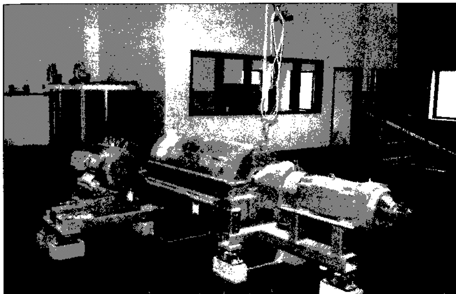
At the Williams Water Treatment Plant in Durham, N.C., a centrifuge is used to dewater the sludge mechanically.
