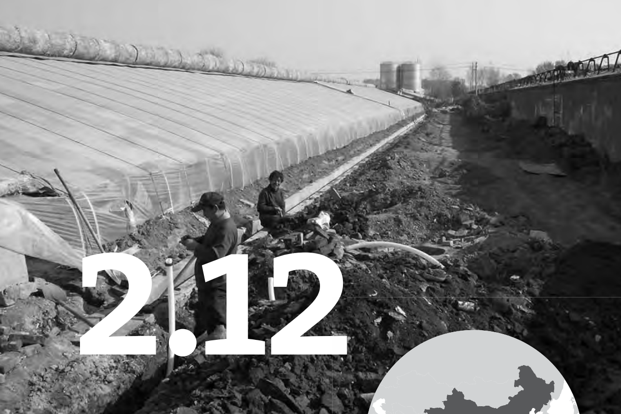
Demonstration site on rainwater harvesting for urban agriculture. (Photo credit: René van Veenhuizen)
