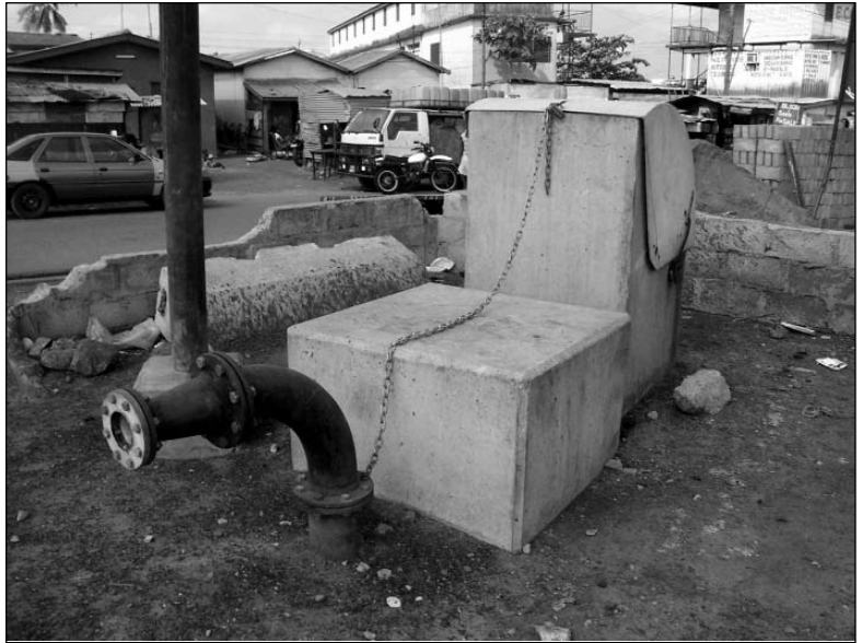
Top of an underground holding tank, showing a chain to lock the lid, a vent pipe and a wall to prevent overflowing excreta travelling onto the road'
