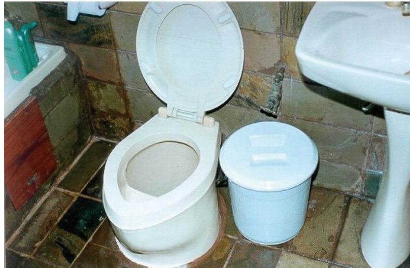
Figure 2.23: Retrofitted urine-diversion toilet in Richard Holden's house in Bellevue, Johannesburg (Photograph: CSIR)
