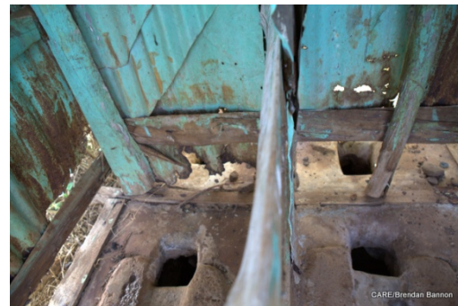
Dirty and deteriorating school latrines. Latrine cleanliness and quality are important for use.
