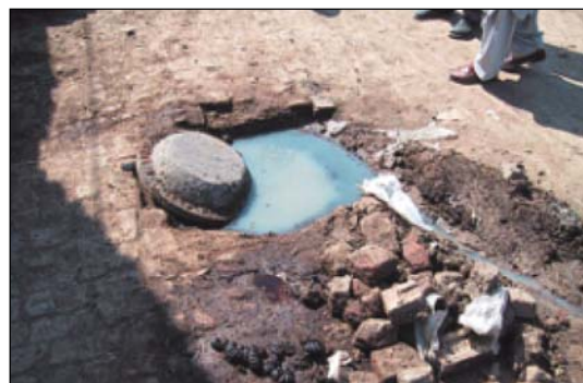
Figure 4-1 Overflow of sewage from blocked sewer
