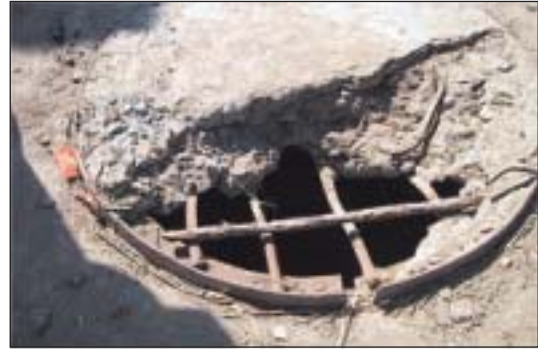
Figure 2-9 Structural decay of manhole cover
