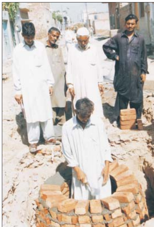
Photo: Some of the community members insisted on manholes constructed with bricks
