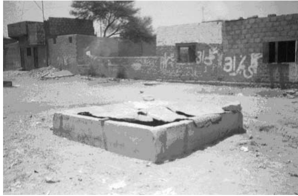
Photograph 5.21. An awami tank at Christian Mohalla, Ghaziabad, Sector 1½, Orangi Town. The tank is covered with broken sheets and gets polluted with dust and other impurities. The physical surroundings are a hazardous situation.
