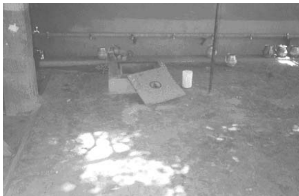
Photograph 5.8. Internal view of an awami tank in Ghaziabad.
