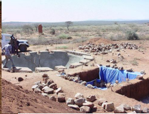
Run off water collection left: using foil (Tunisia); right: in Borana, South Ethiopia (Rain Foundation). Mind sand traps and half circle reservoir
