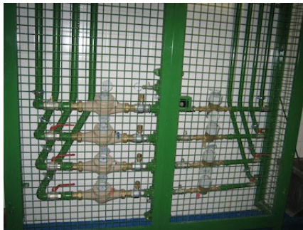
Water sectioning system used in a shopping center.
