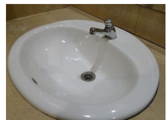
A user-activated automatic shut-off tap system.
