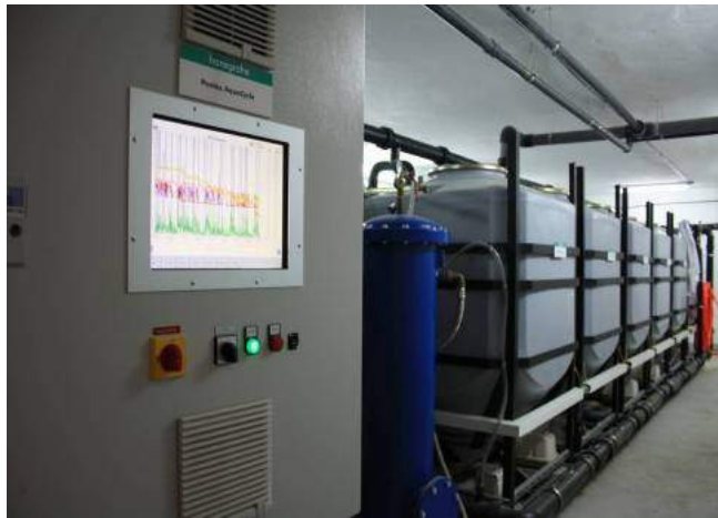
Greywater recycling system.
