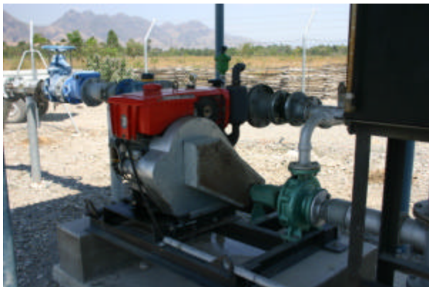
Pump and Motor at Oecussi Bore
