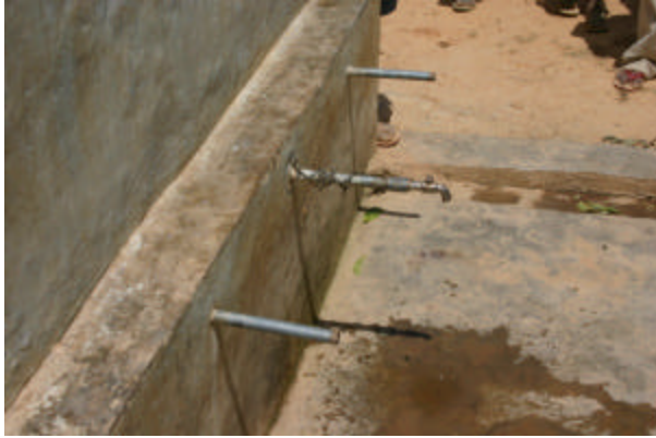
Community-Managed Scheme Missing Taps, No Water
