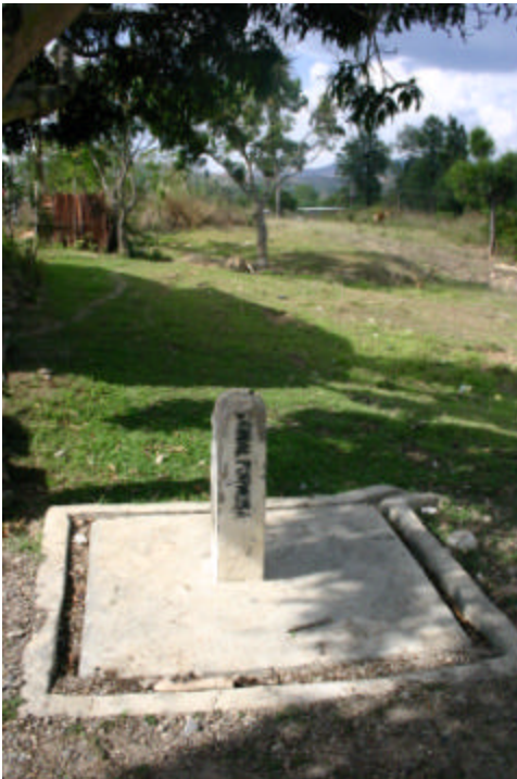
Community-Managed Scheme Vandalized Tap Stand
