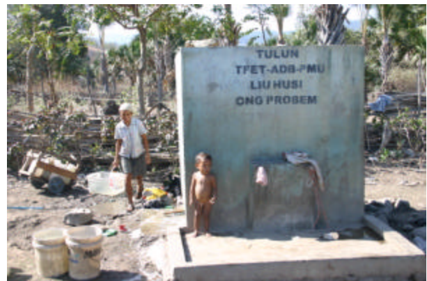
Community-Managed Scheme Non-Functioning Tank and Tap Stand. Pipe Cut to Access Water
