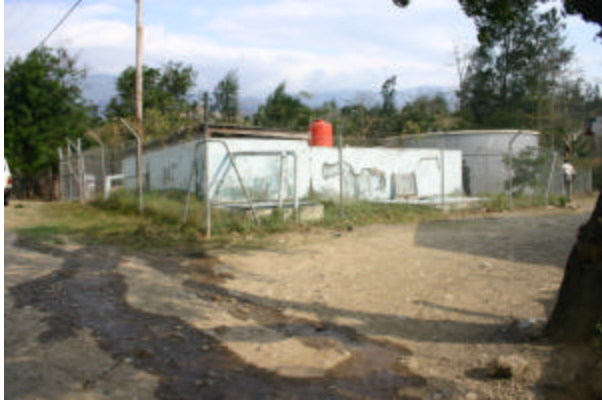
Leaking Storage Tank, Maliana
