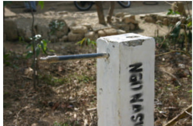
Community-Managed Scheme Missing Tap
