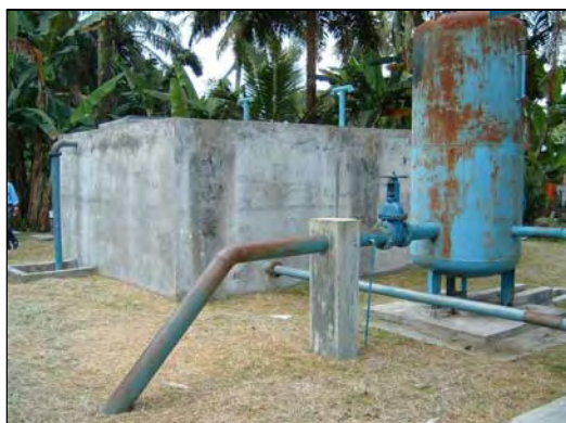
In-line stabilization vessel
