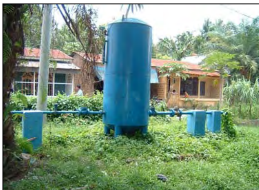
In-line stabilization vessel
