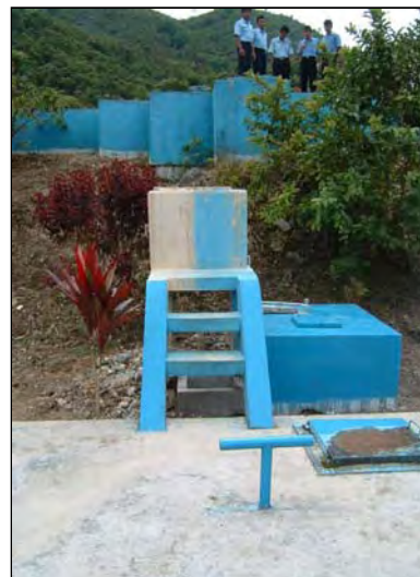
Chemical dosing facilities
