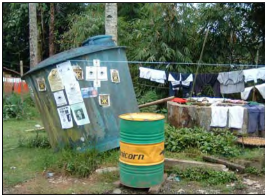
Abandoned public hydrant
