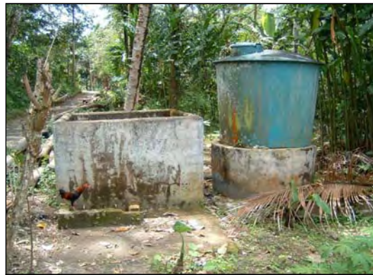
Abandoned public hydrant
