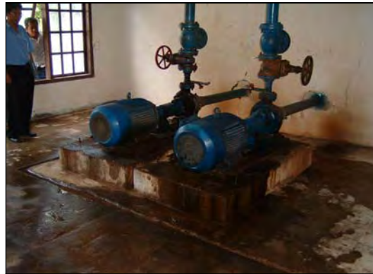
High-lift pumps—pump on the left not working
