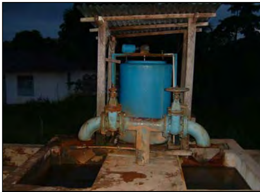
Chemical dosing facilities
