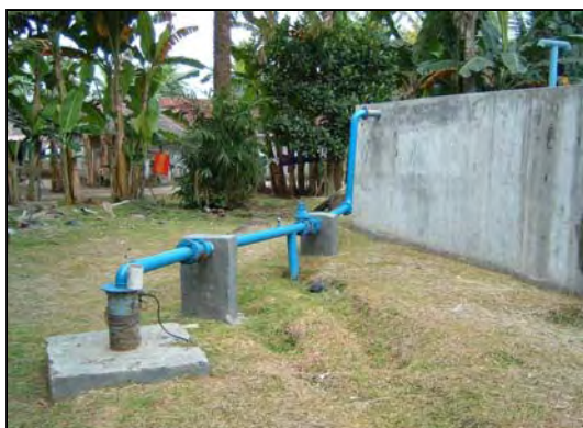
Borehole and header tank
