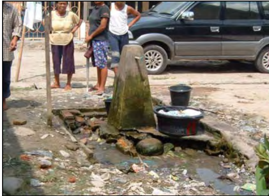
Public hydrant with poor surround
