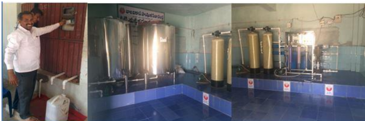
Photograph Bala Vikasa RO unit, with stainless steel water tanks.
