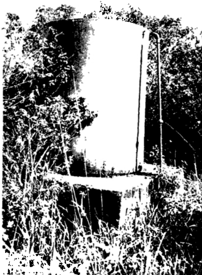
Figure 5. An abandoned storage tank of a piped water supply scheme constructed by a county council in Busia District.
