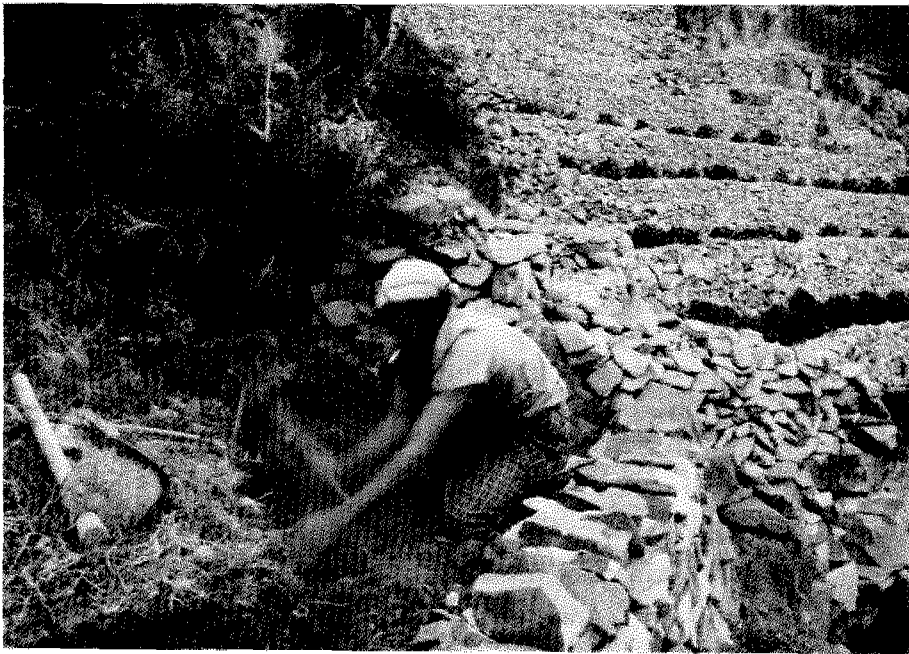
Terrace maintenance will remain an important issue in view of the labour shortage that may become more serious again
