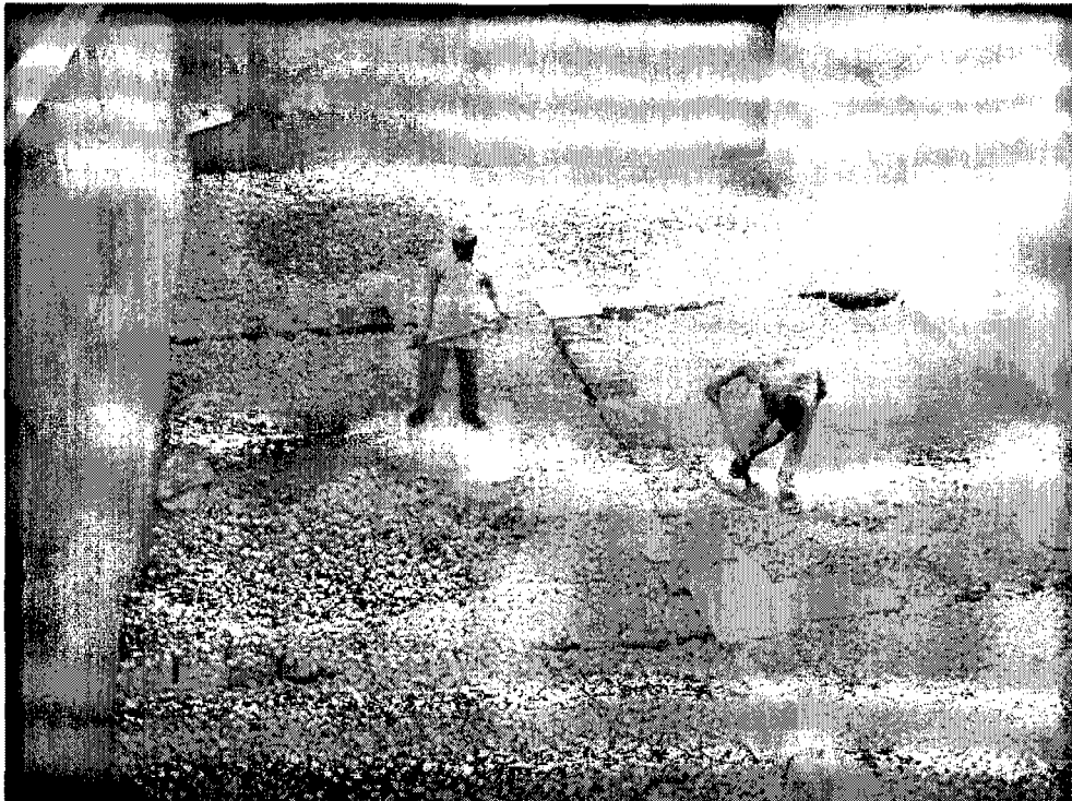
Picture 8: Filter media being filled in Slow Sand Filter
