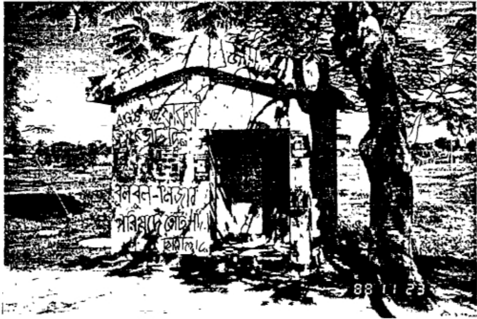
Heavy and costly superstructure to accommodate "demonstration latrine" for use by police in Tangail.
